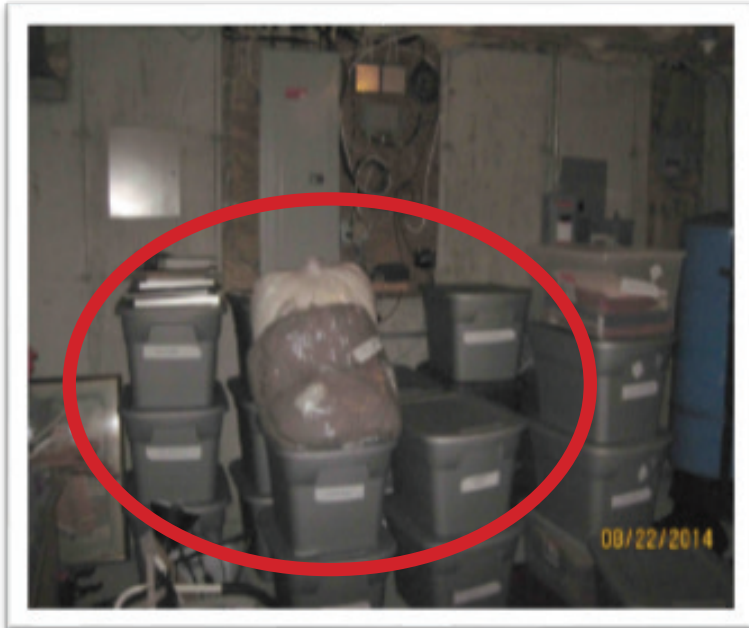
Photo D3: Working clearance not maintained: NEC 110.26
